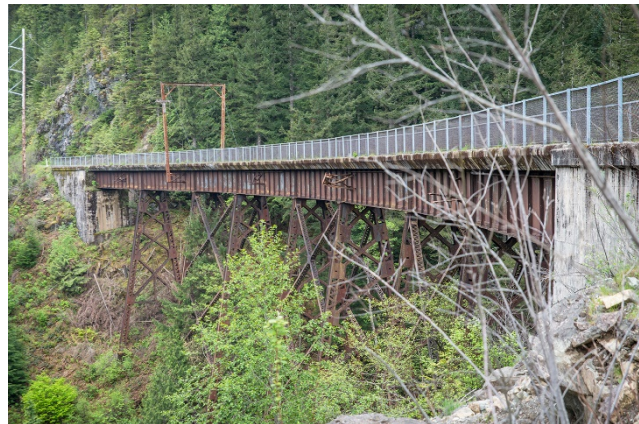
The re-named Palouse to Cascades State Park Trail includes numerous former railroad trestles.
